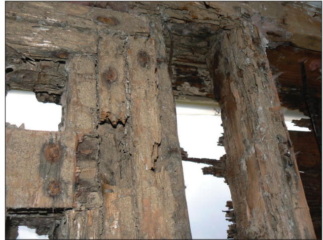
Termite damage to an existing structural bridge member.
