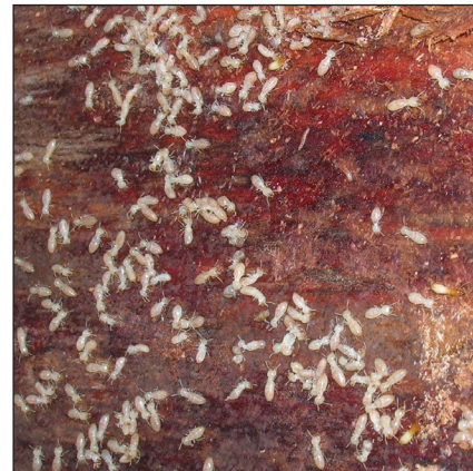
Workers of subterranean termites under the bark of an infested support member.
