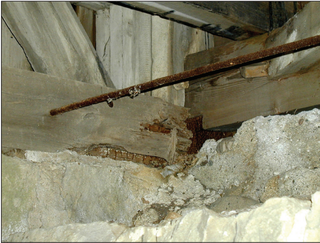
Cubicle brown-rot decay and termite damage to the support members masonry contact under covered bridge.
