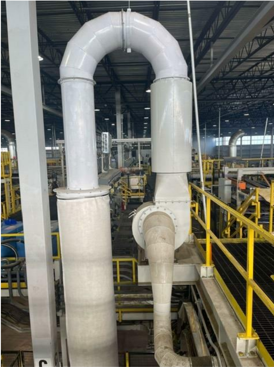
Layup Line #1 Blower/Sock Connection Point
