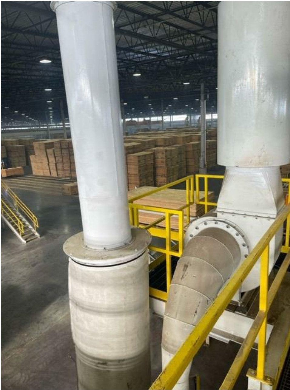
Layup Line #2 Blower and Sock Connection Point
